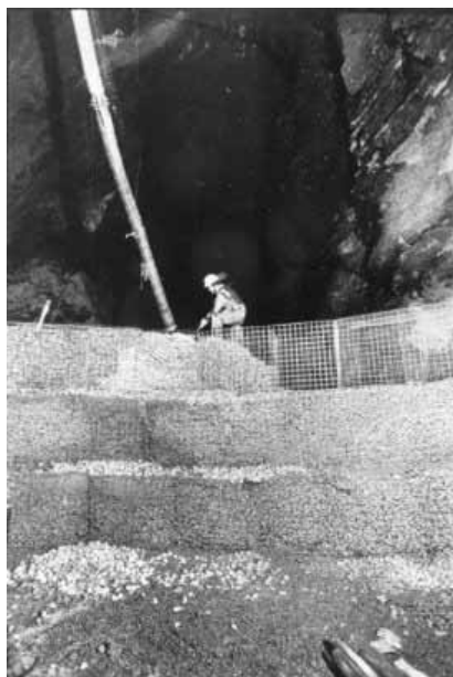
The building of a gravel dam by Groundworks in the limestone caverns
