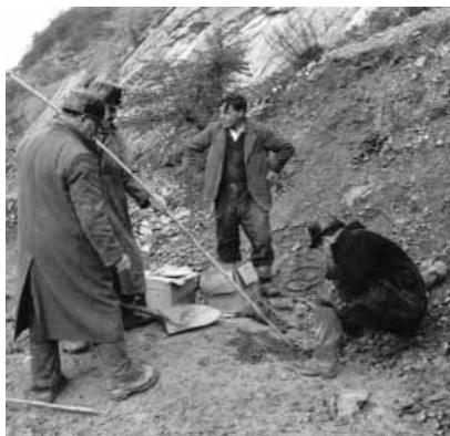
Packing dynamite prior to exploding unstable limestone pillars at the Wrens Nest
